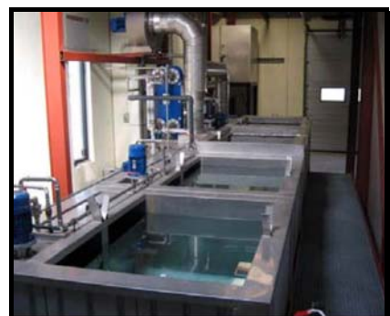
Zinc phosphating facility at Accoat
